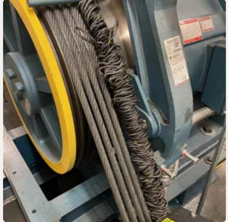
➤ The rope keeper interferes with the running clearance of the traction rope due to an issue with the keeper bracket setup
