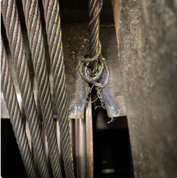
➤ The broken elevator rope that caused the outage
