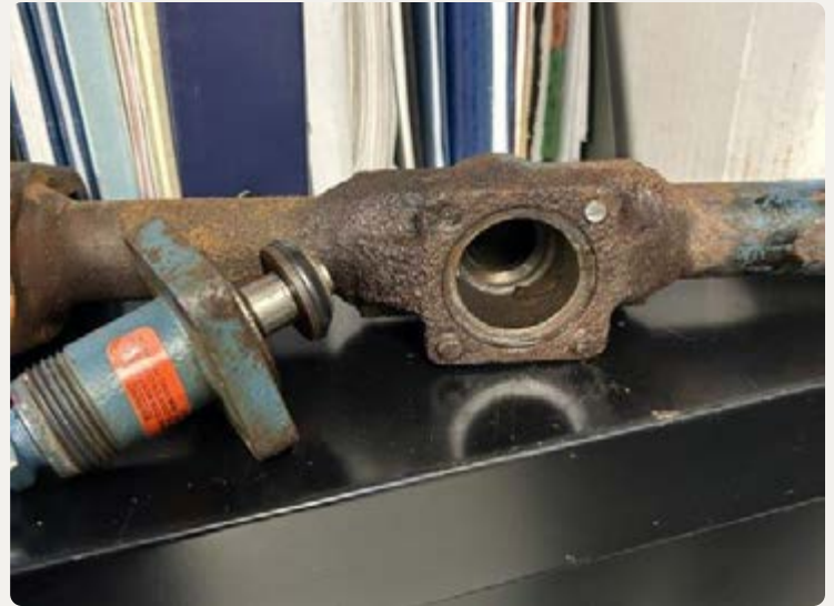
➤ The corroded shut-off valve from which ammonia gas leaked
