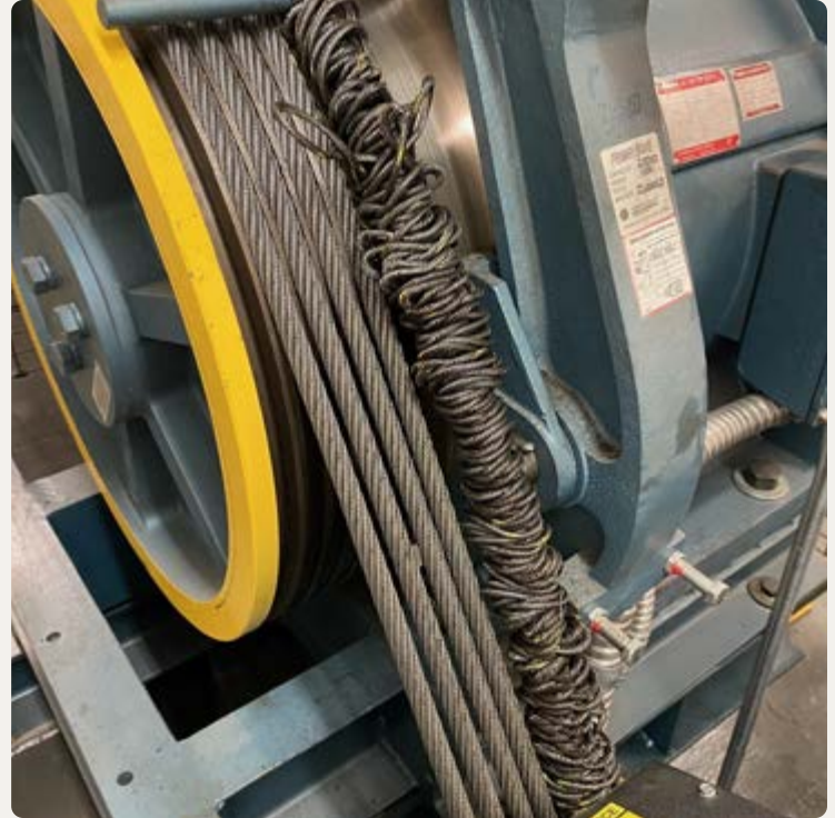
➤ The rope keeper interferes with the running clearance of the traction rope due to an issue with the keeper bracket setup
