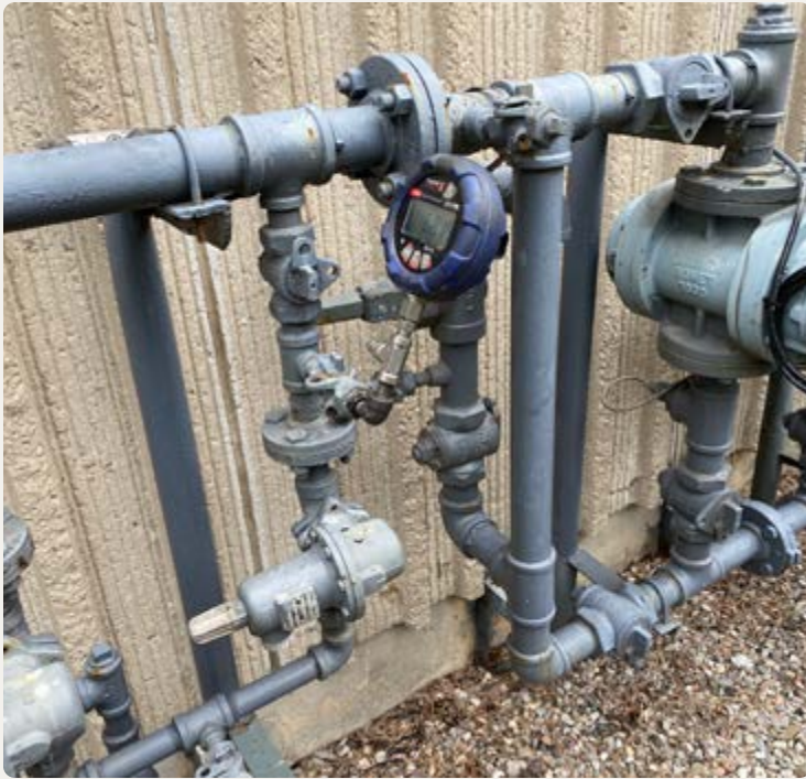
➤ The utility meter that was tampered with by an unauthorized individual
