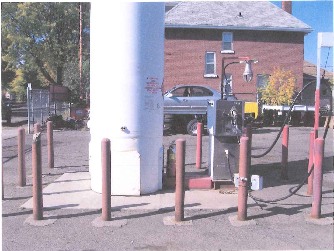
Propane tank Safety Signage Propane tank barriers surrounding it Night Lighting for Propane fuel up with safety lights.
