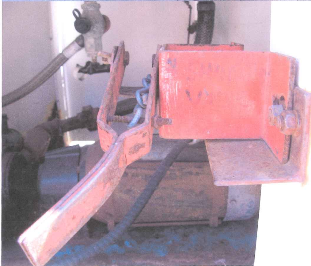
Emergency Shut off Valve door on Propane Storage Tank In order to shut off propane to tank, lift lever up to release chain.
