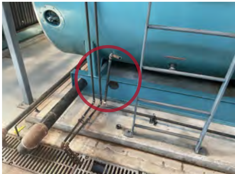
Figure 11: Pipe (indicated in red) was initially lying down and pointing towards the water drain
