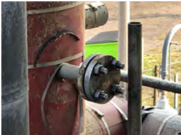
Figure 8: Pressure vessel flange from which ammonia leaked
