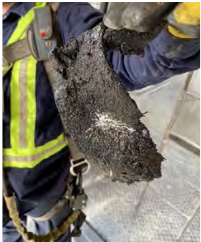
Figure 16: Rigid insulation found in drive pinion
