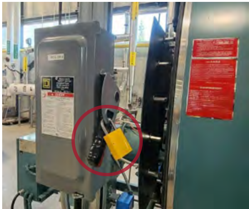
Figure 12: Junction box that powers the boiler locked indicating it is not safe to use
